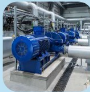
INDUSTRIAL WATER PUMP
